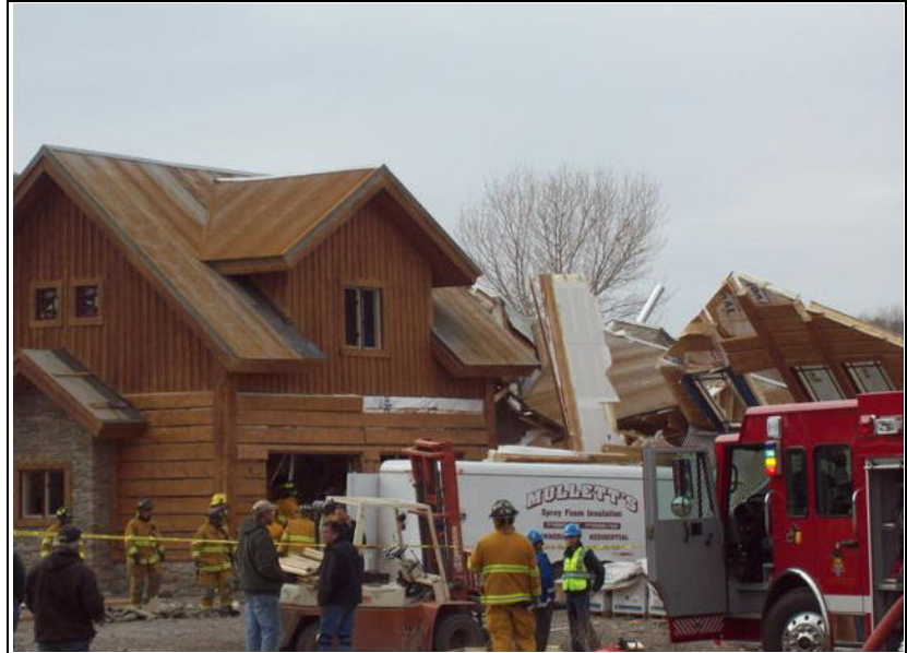
A home under construction exploded in south central Colorado Tuesday afternoon sending eight workers to the hospital with serious burn injuries. (Valley Courier)
